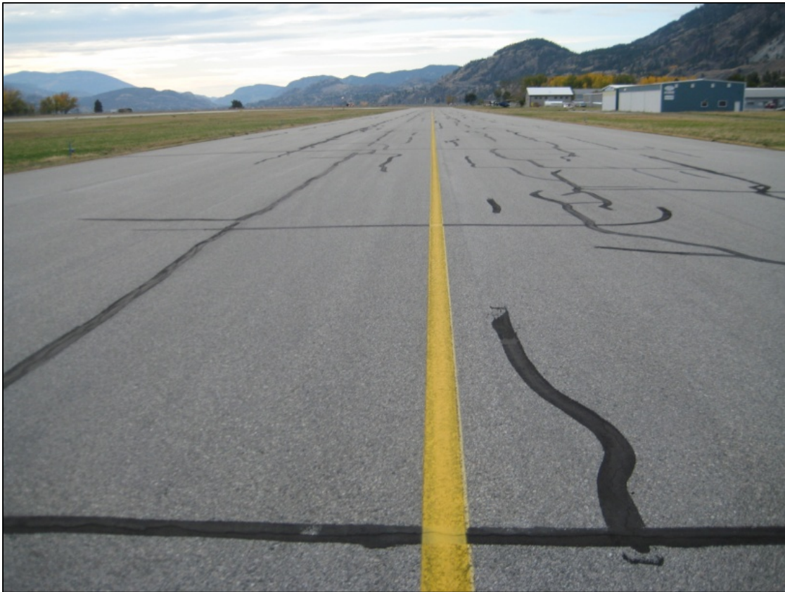
Figure 3. Stand-alone Hot In-place Recycled Surface - Taxiway A at Penticton Airport at 17 Years
