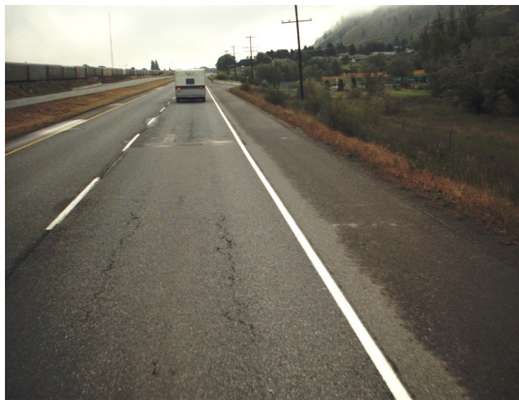
Photograph 2. Pavement surface exhibiting wheelpath cracking and rutting in the eastbound slow lane at Station 14.37.
